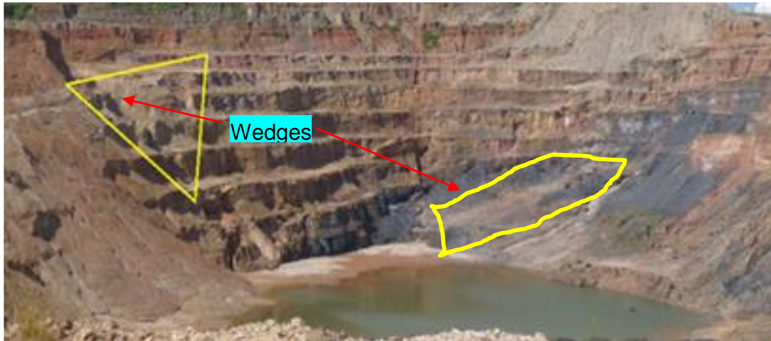
Wedge failure induced by the presence of groundwater at (COP F&D).
